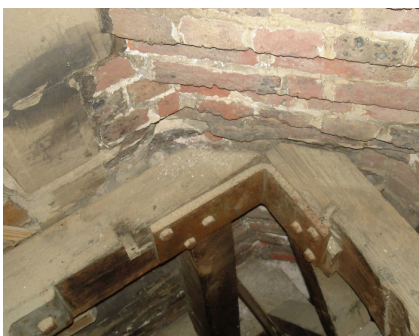
Blackbourn angle bracket compensating for missing corner joint.
